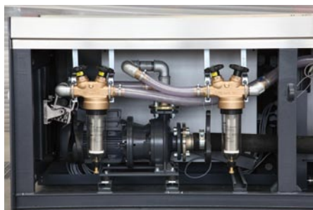
water circulation pump
